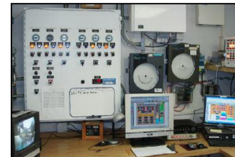
Water plant control room.
